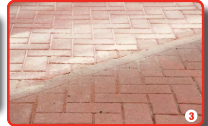
After approximately 1 hour, the surface is set, excess sand is brushed off and the area can be opened to traffic
