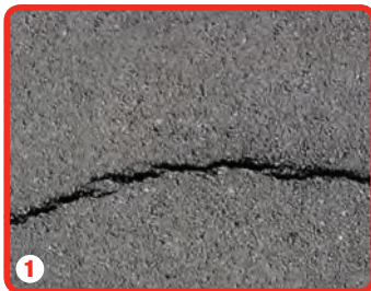
1 Cracks appear in road surface due to heavy trafficking, adverse weather conditions, etc
