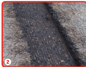
2 Crack is planed out to appropriate width and depth depending on severity
