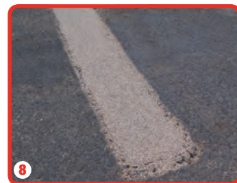
8 Once cured, the excess aggregate is swept clean leaving the road surface safe and secure
